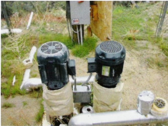
Pressure Pumps at Lower Site
